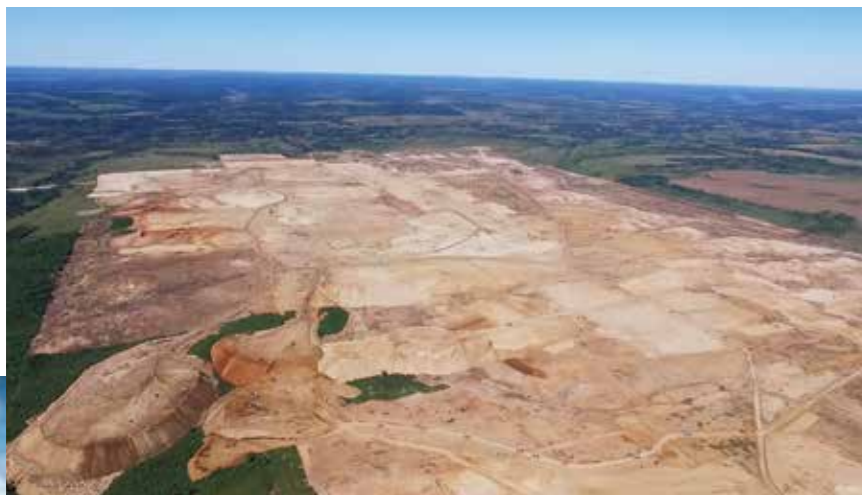
The site for construction and the future project of the Amur Gas Processing Plant
